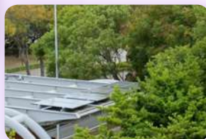
Solar Panels on the Kiln Canopy
