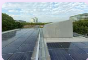
Rooftop Solar Panels on the Story House
